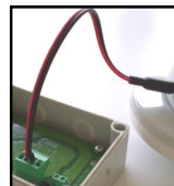
Picture 7 - An example of cable connection between the programmer and a conventional zone module
